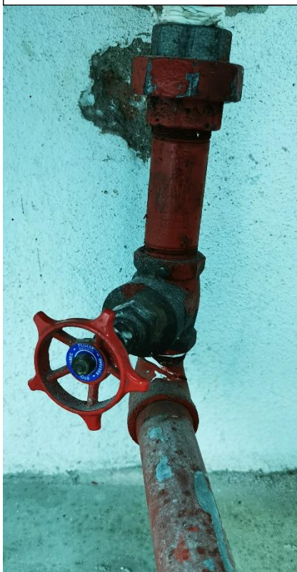
Hand Valve – Hose Reel
